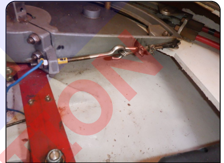
Photo 87: Cable tensioner for steering quadrant
