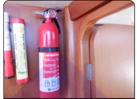
Photo 9: ABC Fire Extinguisher
