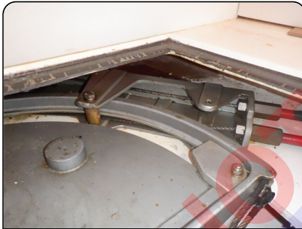
Photo 85: cables to steering quadrant
