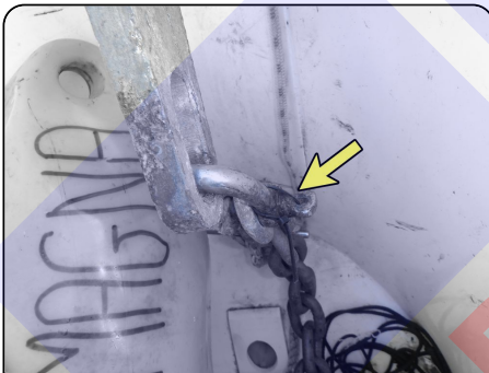
Photo 28: No safety wire just a zip tie
