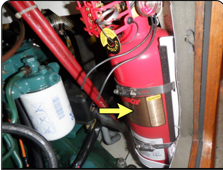
Photo 14: fireboy automatic fire extinguisher
