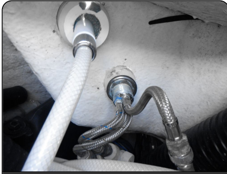
Photo 23: Aft deck shower water lines
