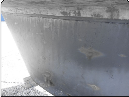
Photo 136: Keel exposed and rusting
