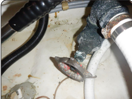
Photo 115: Valve for overboard discharge.
